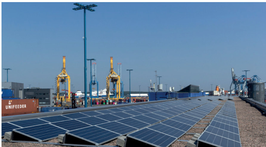
Solar panels installed on the office roof have provided renewable electricity for about six years. Photo Catarina Stewen
