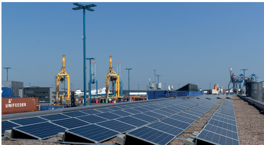
Solar panels installed on the office roof have provided renewable electricity for about six years. Photo Catarina Stewen
